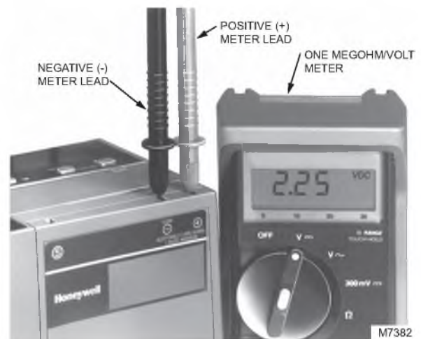
Fig. 5. Measuring flame signal voltage of 7800 SERIES controls.
