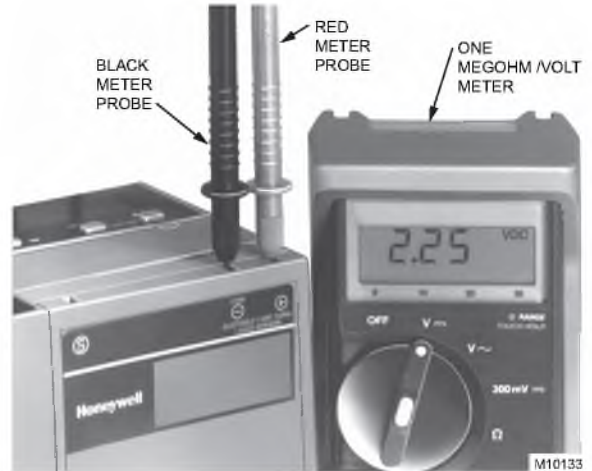
Fig. 11. Measuring voltage flame signal with 7800 Series controls.
